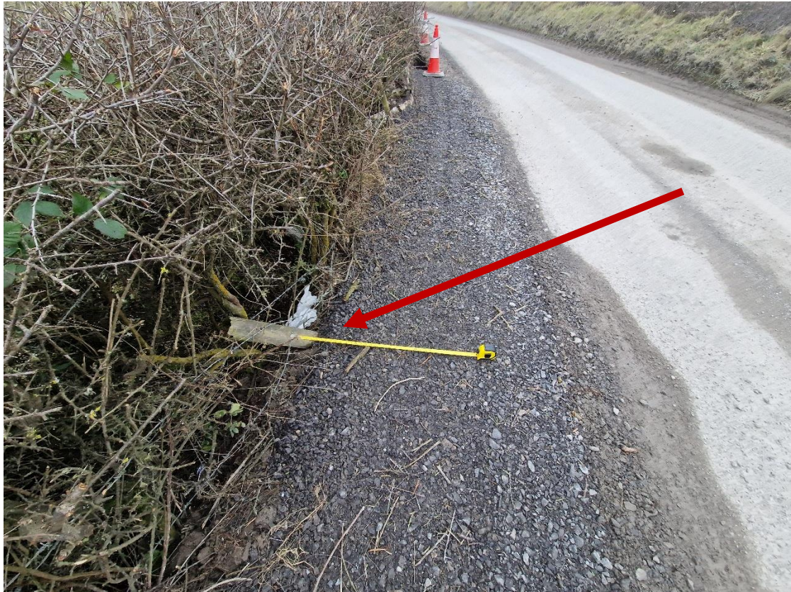
Figure 38: Encroachment onto my property, damage to roadside hedge and flattening of barbed wire fence (arrow shows previous upright fence post flattened and partly covered by road filling) January 2024
