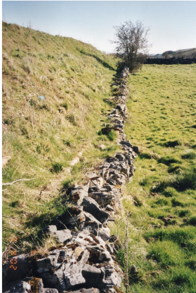
Figure 29: Partial collapse and push-back of our drystone walls caused by McCaffrey's creation of the berm (pictured in 2002, looking north-eastwards). Machinery yards are now located on the other side of this berm to the left.
