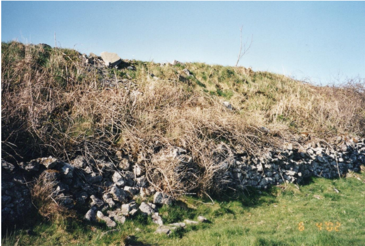
Figure 30: Damage to our drystone walls along the boundary of the South Quarry (pictured 2002) at a location to the west of the road to the quarry. Besides the very significant damage to these drystone walls, it also created the problem for running the farm as McCaffrey's actions resulted in the fields no longer being stockproof.
