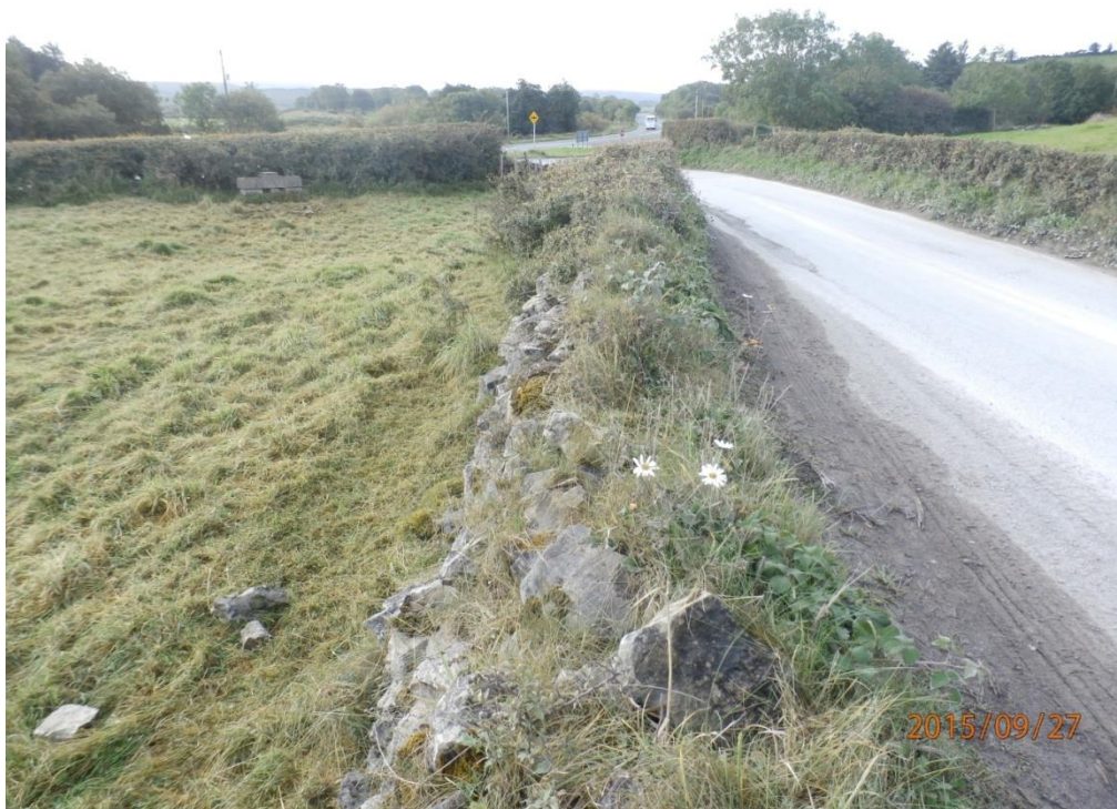
Figure 32: Quarry operator has raised access road by 600mm putting additional weight on drystone field walls
