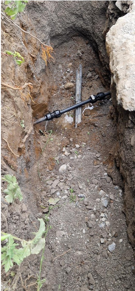
Figure 42: Repair of my farm water supply pipe
